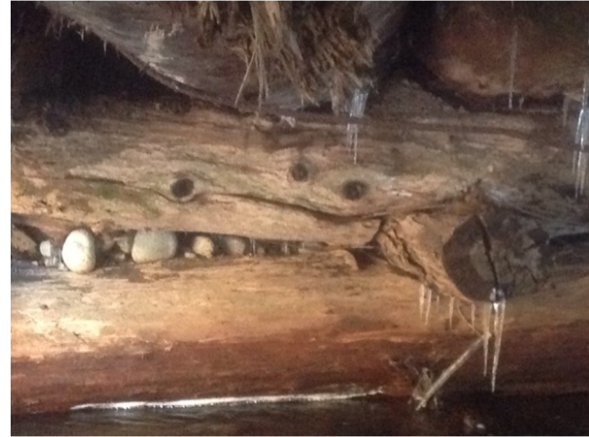
top crib log on left abutment has horizontal crack
